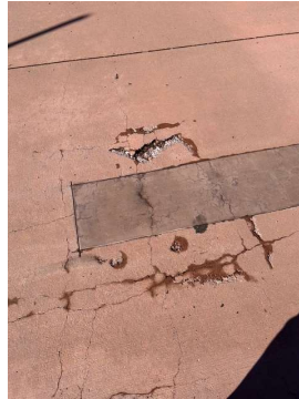
Deteriorating pool deck at Aquatic Center
