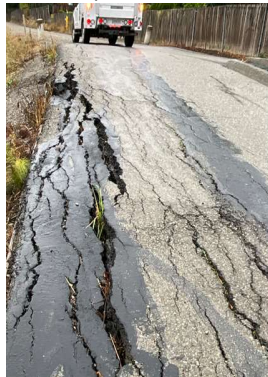
Arroyo Mocho Trail repair needs
