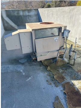
Police Department HVAC installed in 1997
