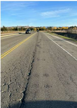
Deteriorating Roadway at Busch Road
