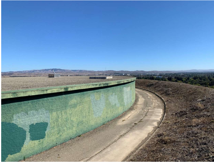
Figure 4 Foothill Water Storage Tank
