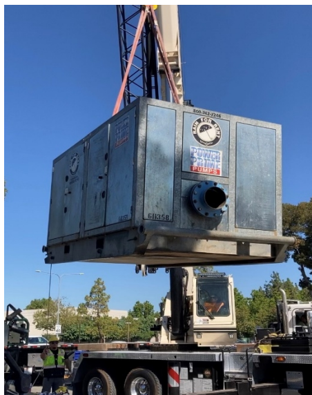
T-4 Temporary Booster Pump
